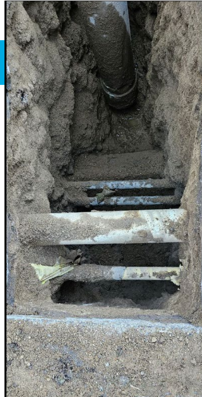
Heating Well Obstructions Identified
