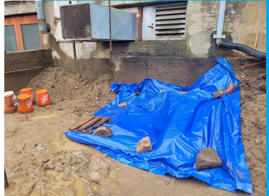
Asbestos area covered by plastic containment (March 2023)
