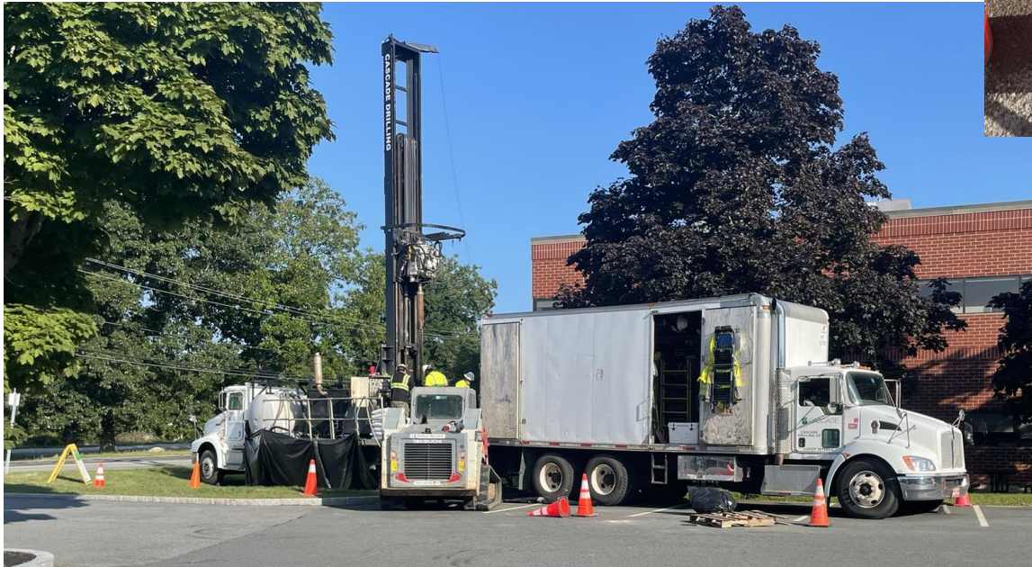
Sonic drilling at 30 Tozer Road to install a nested monitoring well (August 2024)
