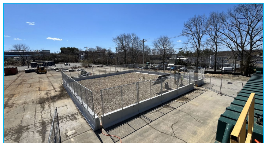
Figure 4. Final SGBR treatment cell.
