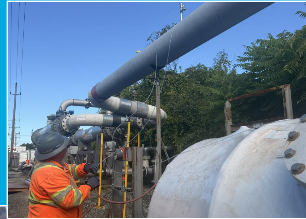
Monitoring thermal treatment system
