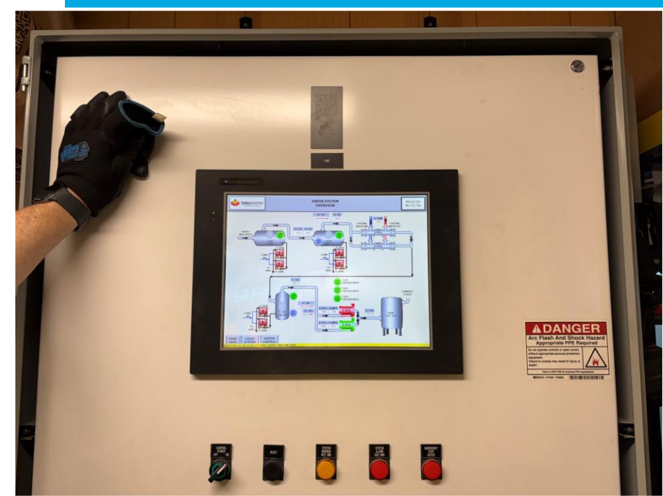
Thermal System Control Panel
