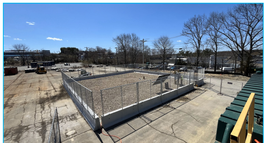
Figure 4. Final SBGR treatment cell
